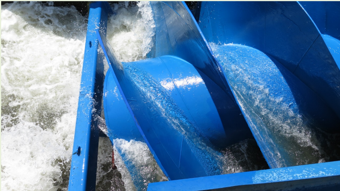
Lower end of the Archimedes screw at the Kuhlemühle power station in the Diemel. Photo by Eva B. Thorstad.
